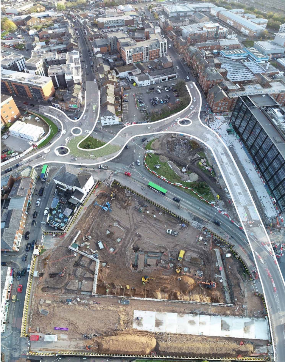
Figure 5. Adelphi Quarter under construction- a sketch of new carriageway layout (©E. Kamel)
