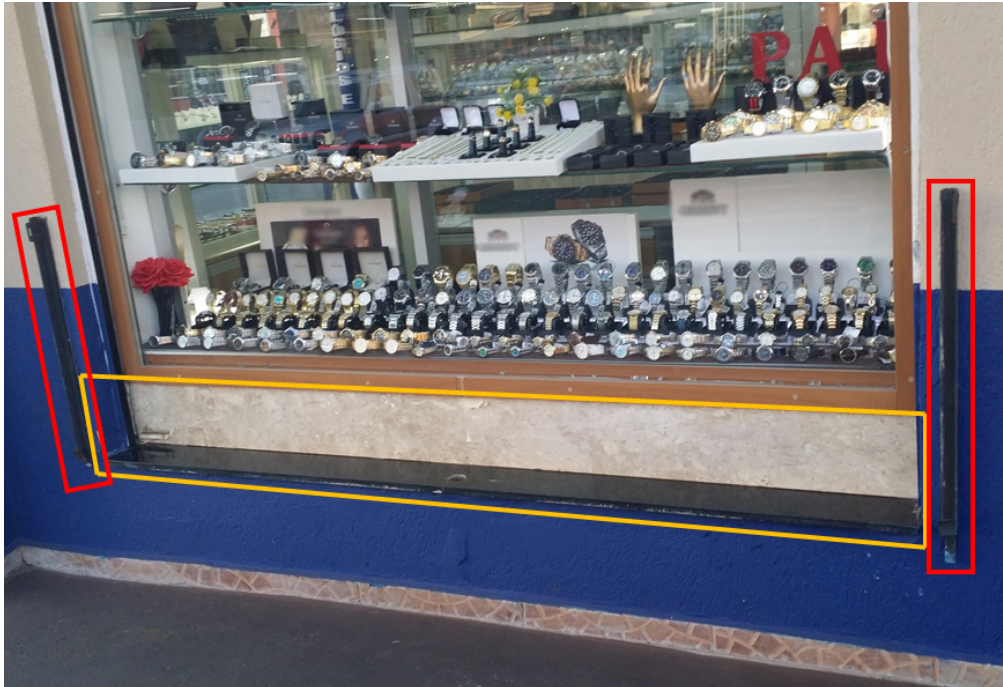
Figure 3: Adaptive measures in a jewellery store in the Municipal Market area. The floor level enhancement is highlighted in yellow, and the supports for the flood barrier are highlighted in red.
