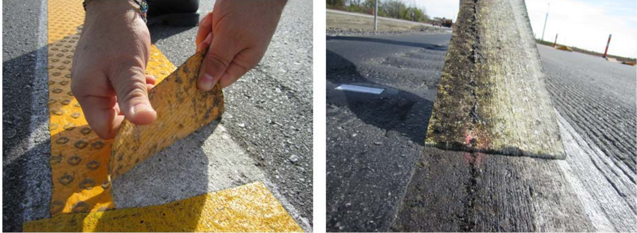
Figure 16. Marking removal from a variety of surfaces
