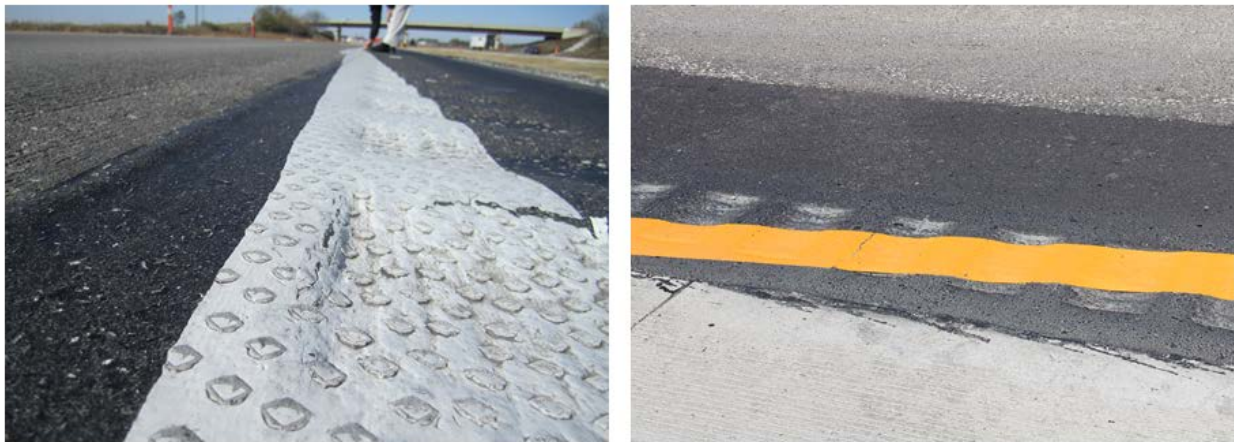
Figure 14. End of project condition for trailing edge-line markings
