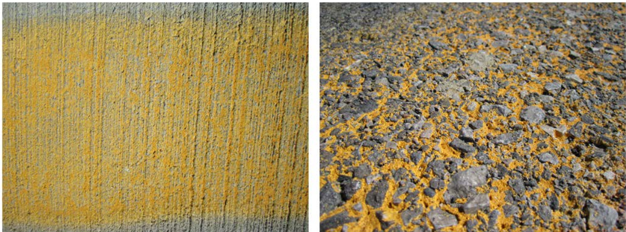
Figure 10. Paint loss (yellow) after 15 days within the crossover
