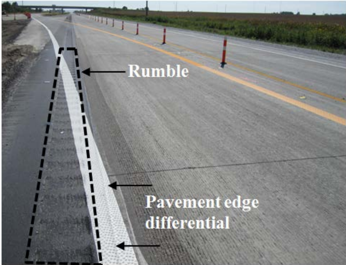
Figure 15. White edge line along the trailing end of the crossover
