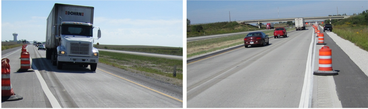
Figure 11. Vehicle lane positioning away from the white edge line within the taper area
