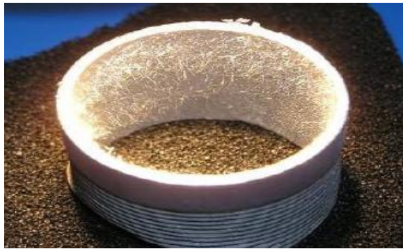
Figure 9.2: Zinc whiskers on a hot dip galvanized steel pipe, Courtesy of NASA
