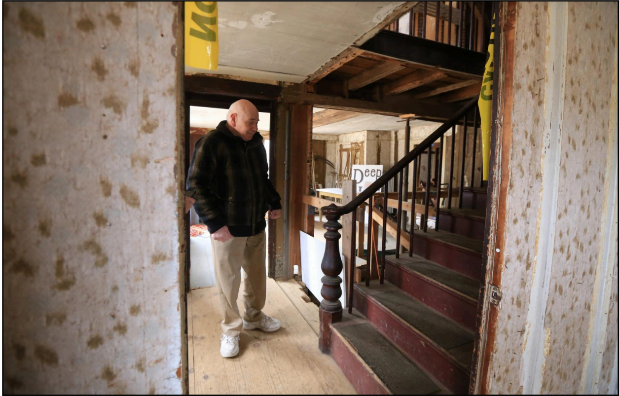
Image 5.8: Skip Webb, president of the James House Museum and Association, standing at the foot of the staircase inside of the historic house. From this image, viewers can see the exposed framing of the first floor, and the former location of the central chimney, now removed. Caution tape is also depicted in this image, noting the numerous safety concerns of the house still under restoration. (Sourced by Seacoast Online 2019)
