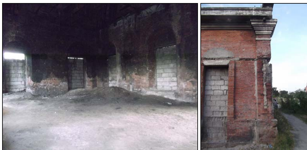
Figure 104 and 105: Interior (left) and exterior (right) damage to the San Fernando Train Station.
