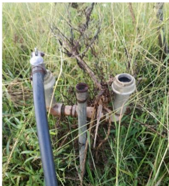
Figure 4.13: Irrigation pipes near Lenye Youth Group plots (1 April 2017)
