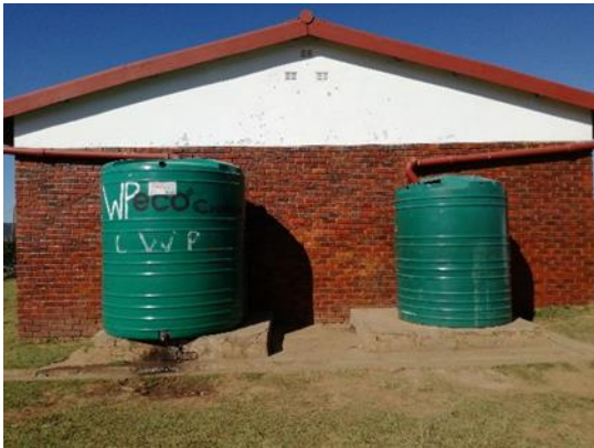
Figure 4.16: Lenye Primary School tanks (17 May 2017)
