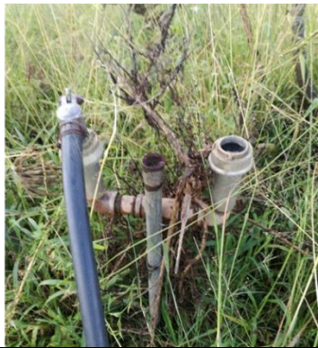
Irrigation pipes near Lenye Youth Group plots
