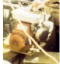
① a pump used to apply wastewater
