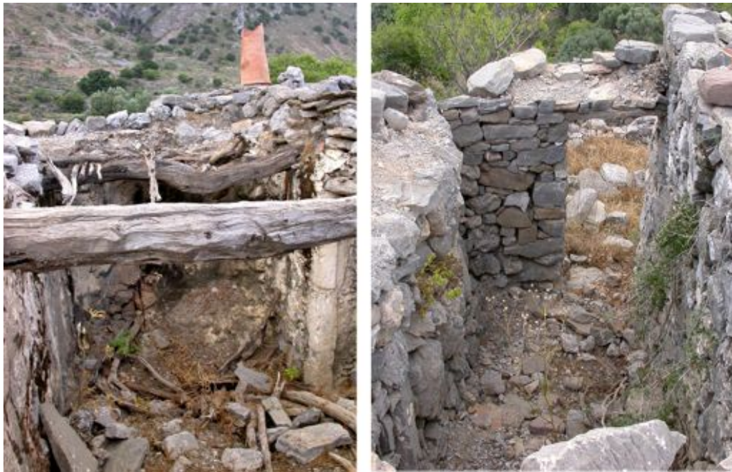
Figure 4: Partially collapsed (modern) field houses near Kavousi, Ierapetra, Crete
