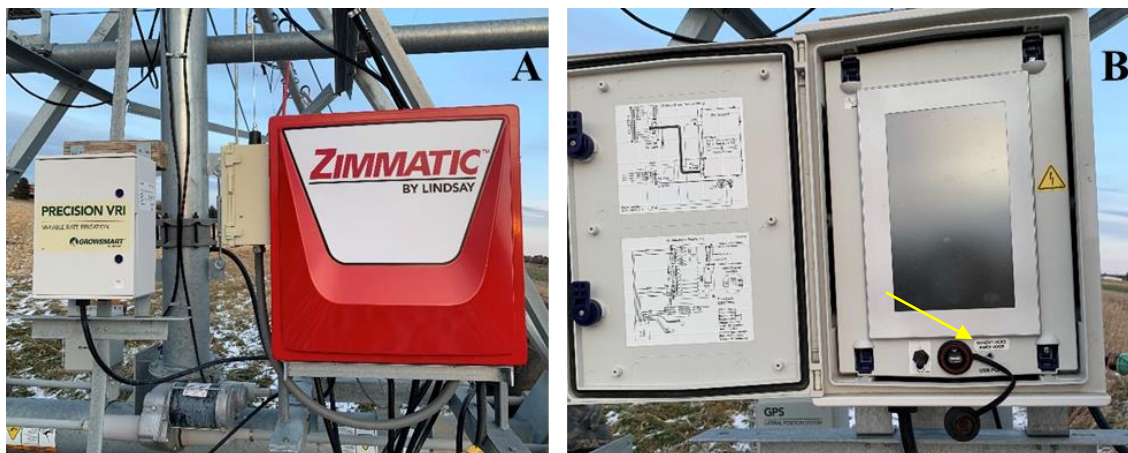
Figure A.6. Precision VRI and linear system control panels (A). Precision VRI box and USB port where irrigation plan is uploaded (yellow arrow) (B).
