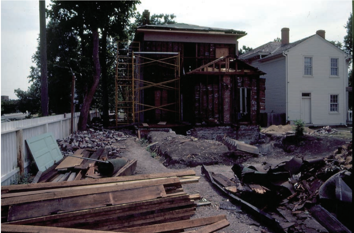
Figure 13. Photo showing the extent of disturbance during the 1979 restoration work in the back of the Beedle house. Courtesy of Lincoln Home National Historic Site Photo Archive Database. http://liho.missouri.edu/Default1.asp . Photo ID B8F12P136
