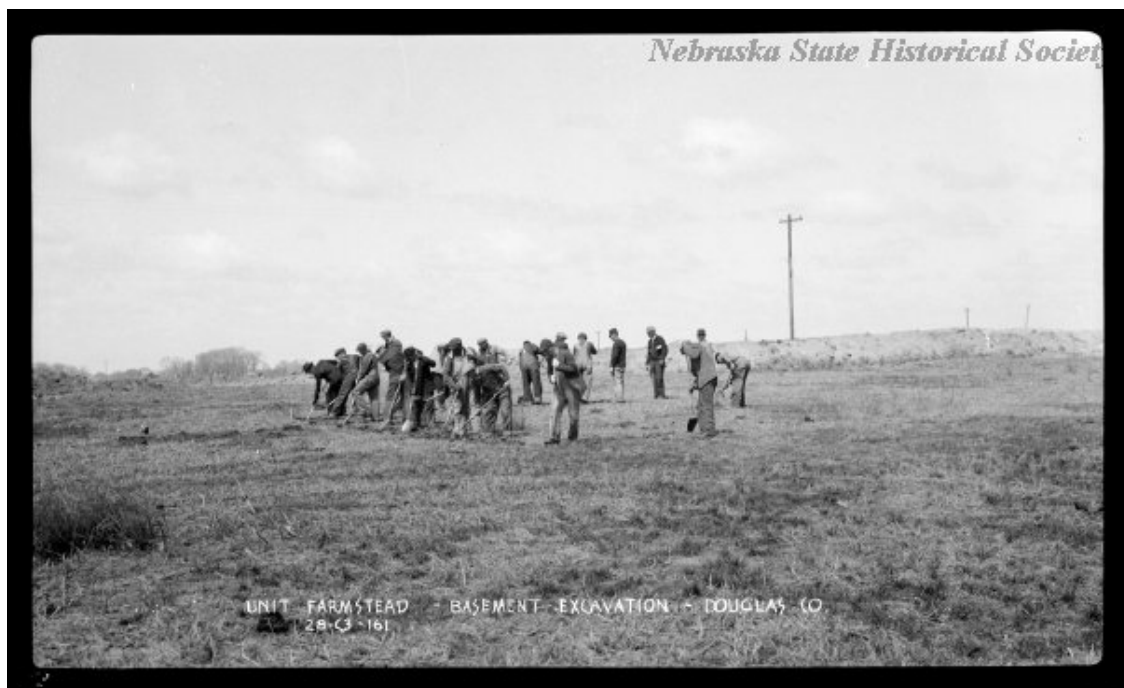
Figure 5.26. Two Rivers Farmsteads, 1935. They were digging a basement for a house by hand (Nebraska State Historical Society).
