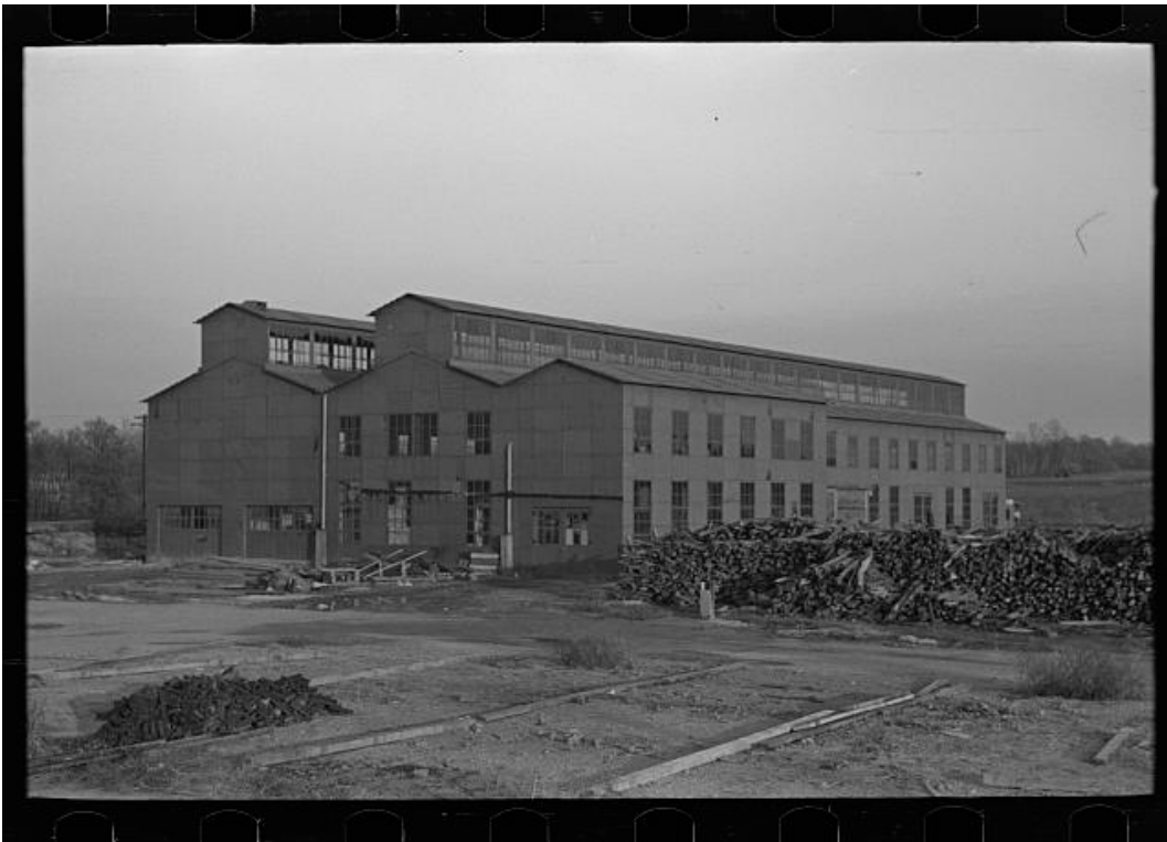
Figure 4.6. The canning facility under construction in Hightstown, New Jersey (United States Resettlement Administration, 1936).
