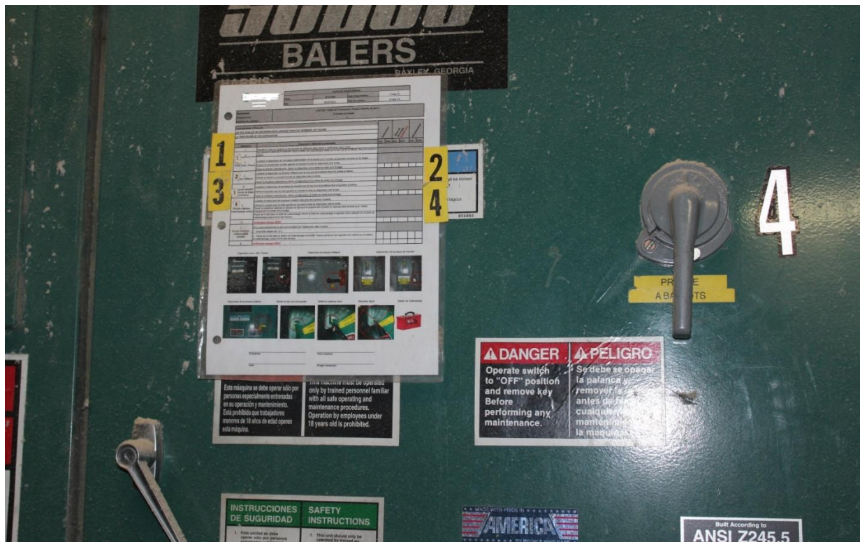
Figure 4-2 Lockout placard posted on a machine
