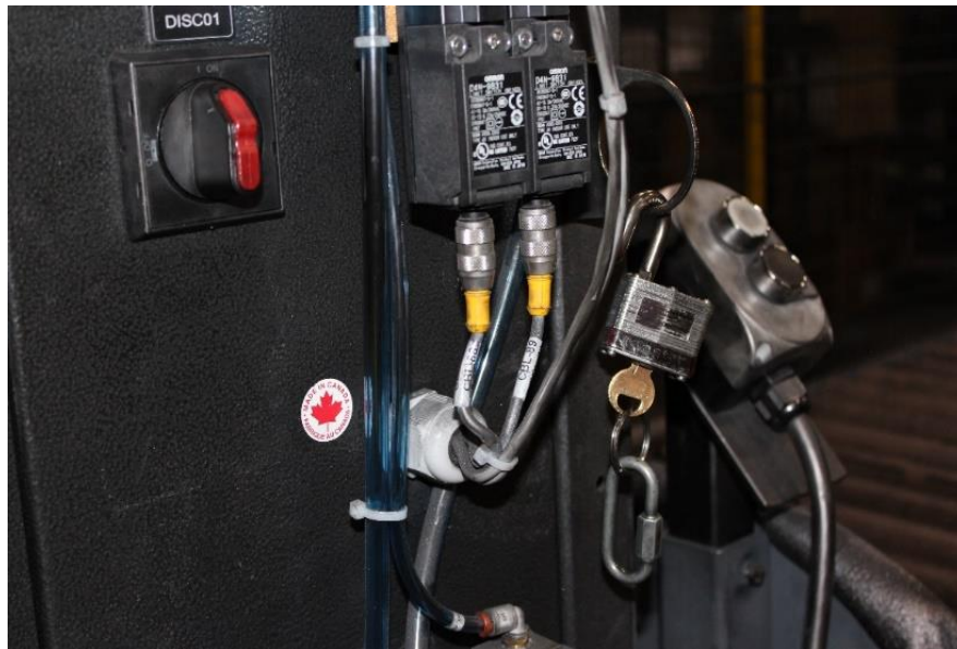
Figure 5-2: Disconnecter with a regular fixed padlock
