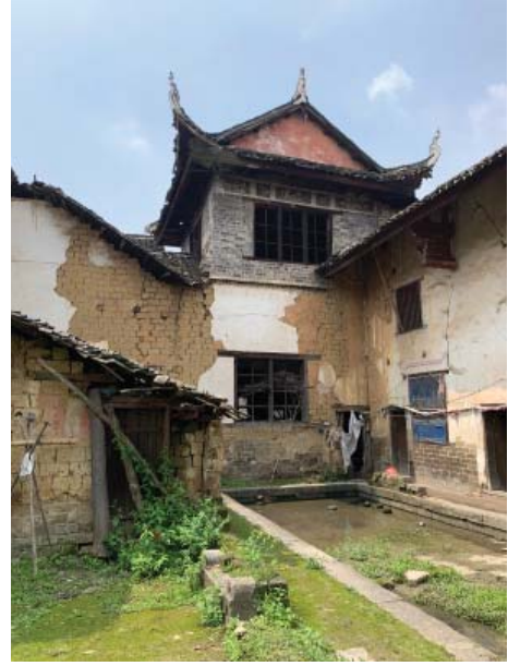
Figure 2.18 Collapsed southern Tian-jing
