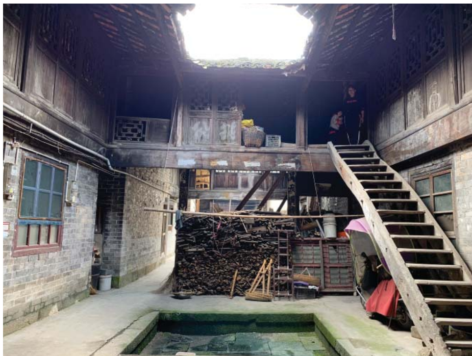
Figure 4.13 Sectional division removed on the ground level. Residents used the left-over space for storage and added stairs to connect to the upper level. The upper sectional division remain as corridor connection for the upper level.
