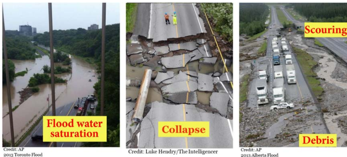
Figure 4.2 Pavement Flooding Damage Pictures
