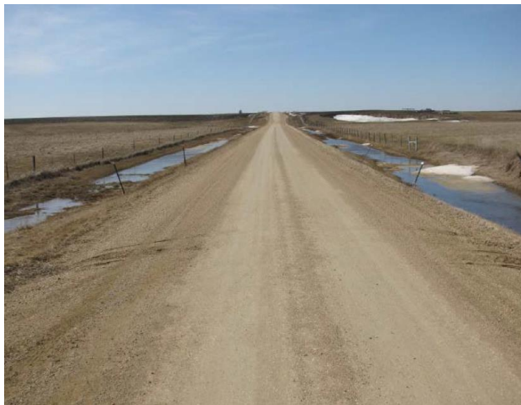
Figure 2.12 Gravel road with excessive crown.
