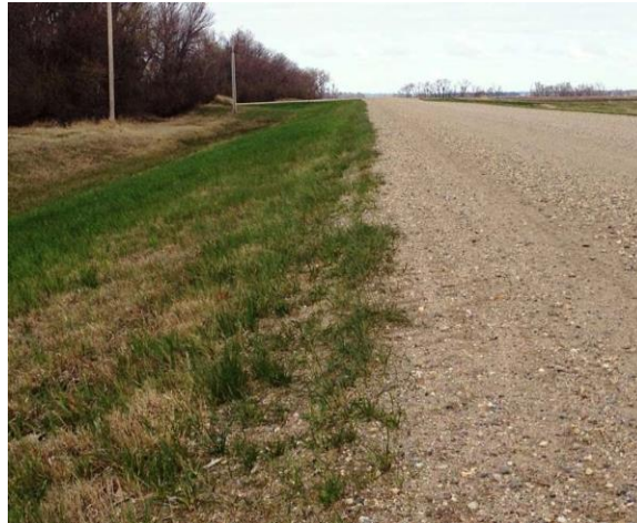
Figure 2.13 Example of good gravel shoulders.
