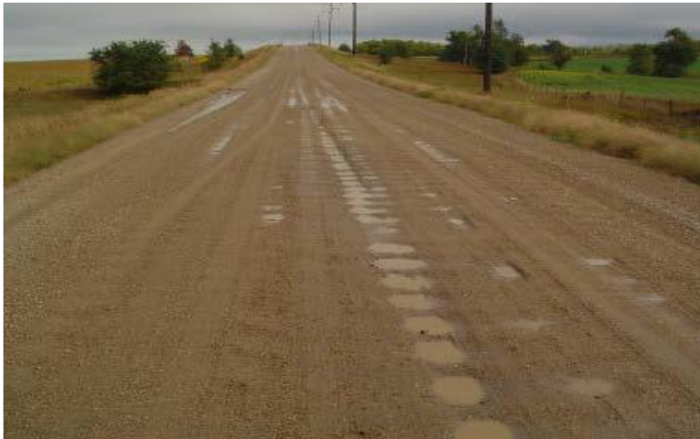
Figure 2.11 Gravel road with inadequate crown
