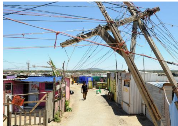
Fig.11: This shows how the typical informal settlement is a mess of exposed electrical cables as a result of cable theft that results in a deadly environment. (Source: https://www.iol.co.za/news/south-africa/eskom-warns-about-dangers-of-electricity-in-rainy-weather-2093095 )
