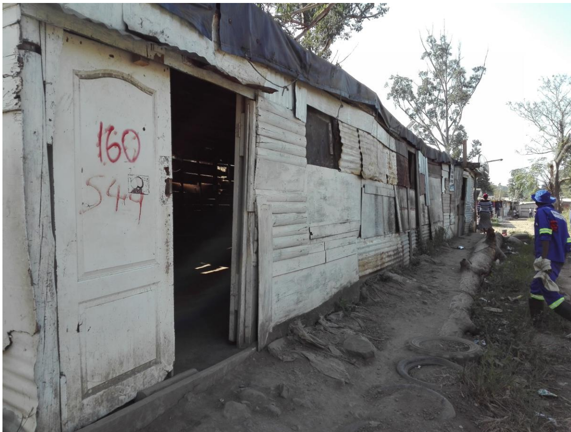
Fig.15: The Church and community hall at the Quarry Road West informal settlement displays an assemblage of materials like wood and scraps of corrugated iron used to clad the timber frame structure. (Source: Author)
