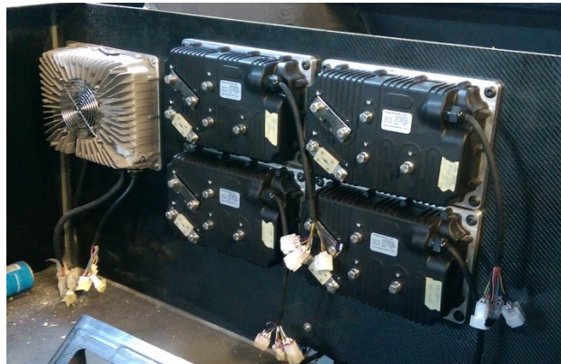
Figure 7-7. Motor controllers and charger mounted on the rear firewall of the Mamba EV.
