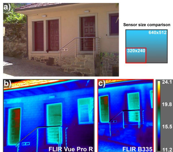
Figure 6. (a) RGB (red-green-blue) images of part of the building and thermograms obtained from the same point (~4 m from the façade) with (b) the FLIR Vue Pro R and (c) FLIR B335 cameras. The same colour palette and ST scale are used. The temperature scale is in °C.
