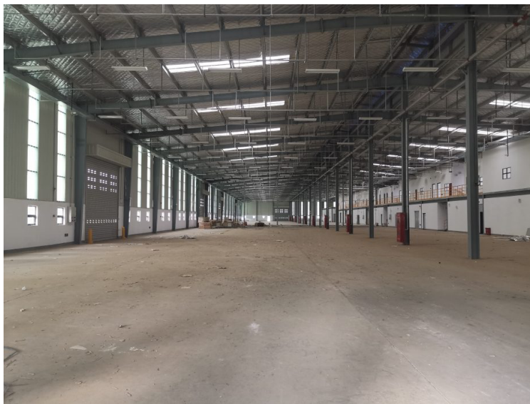
The inside of an empty shed in Mekelle IP. Credit: Istvan Tarrosy
