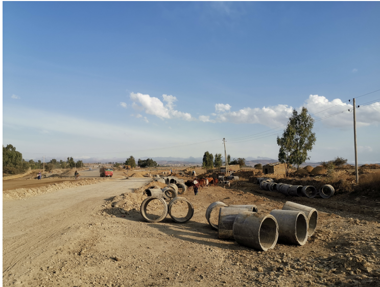
Ongoing road construction work, three years after the IP's inauguration. Photo by Istvan Tarrosy.
