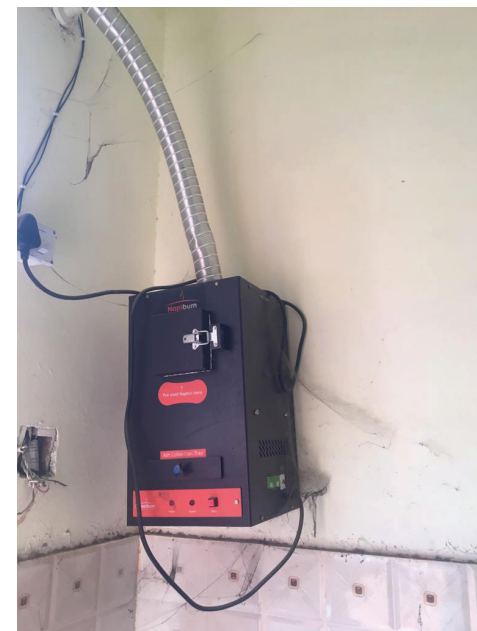
Image 43. Small-scale incinerator inside the washroom for burning pads
