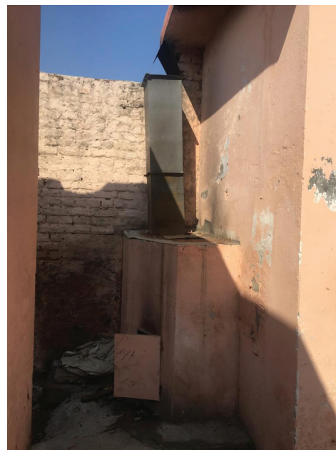
Image 42. Chimney outside washroom to burn menstrual waste
