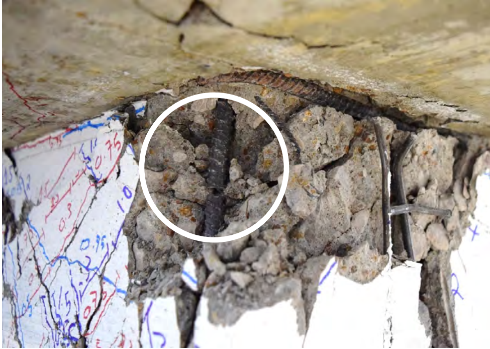
Figure B.26 – CB2D with longitudinal bar fracture during second cycle to +5% chord rotation
