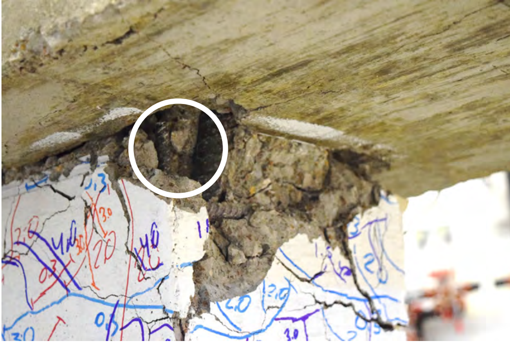
Figure B.21 – CB1 with longitudinal bar buckling during first cycle to -5% chord rotation
