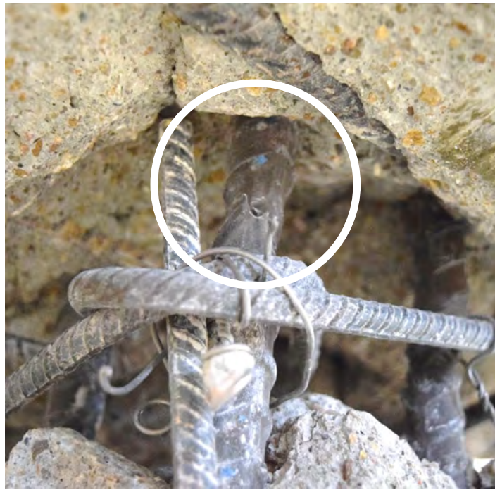
Figure B.25 – CB2 with two diagonal bar fractures during first cycle to +6% chord rotation
