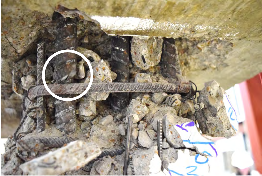
Figure B.23 – CB1 with diagonal bar fracture during first cycle to +8% chord rotation
