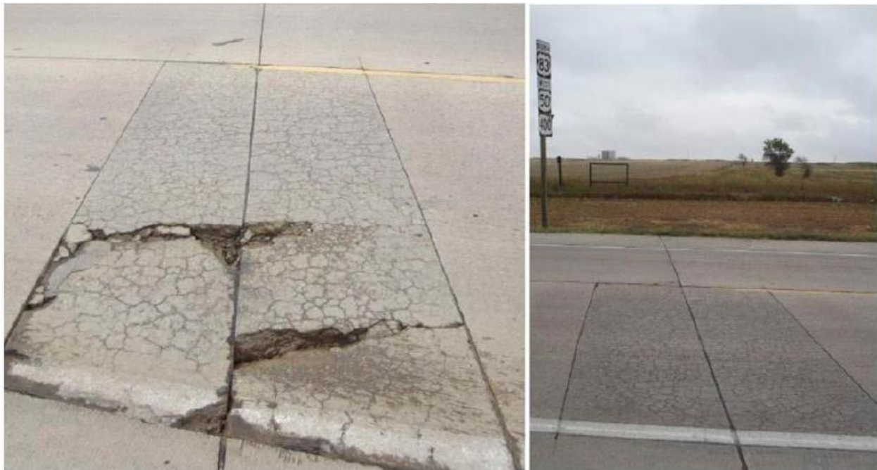
Figure 1-1: Prematurely Deteriorated Slabs in Garden City, Kansas
