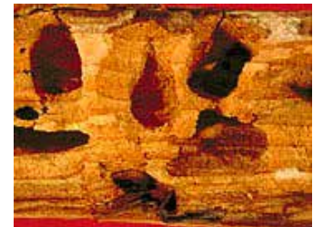
Carpenter ant galleries (close up)
