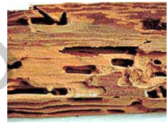
Carpenter ant galleries
