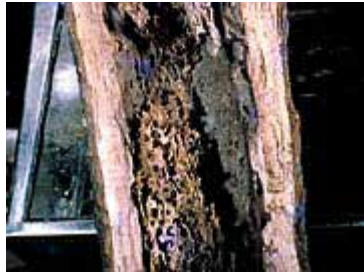
Carpenter Ant damage
