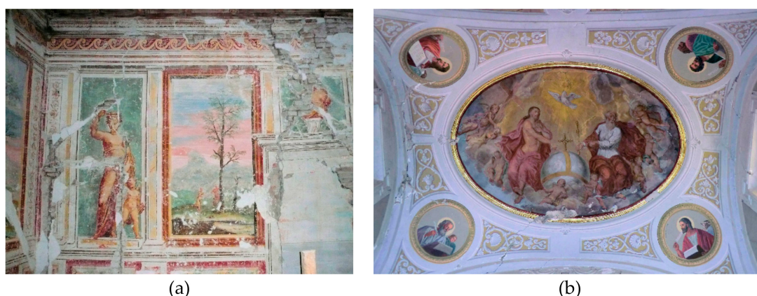
Figure 5. Example of primary and secondary mechanisms associated with a damaged fresco located in apse of a church: (a) apse is subjected to ‘overturning’, but the main mechanism affecting fresco is ‘shear’; therefore, ‘in-plane mechanism of apse’ and ‘overturning of apse’ are, respectively, primary and secondary mechanisms; (b) damage to the vault of the central nave affects the painting as a primary mechanism.
