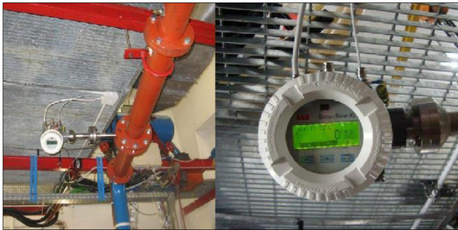
Fig. 2.18 – ABB Sensyflow FTM500-IG Installed on Testing Line
