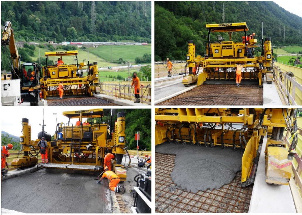
Figure 1: Switzerland 2018 [12] - Retrofitting of a bridge deck member by using a commercial UHPFRC
