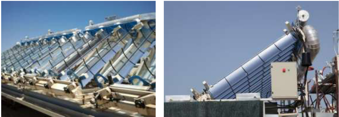
Fig. 10: View of the demonstration site in Malta, installed by Arrow Pharma company
