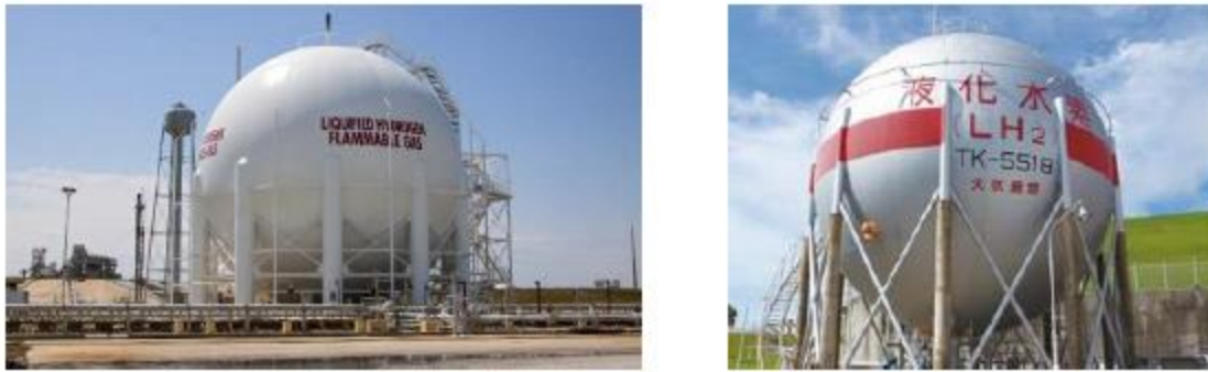
Figure 13 Liquid hydrogen storage tanks.
