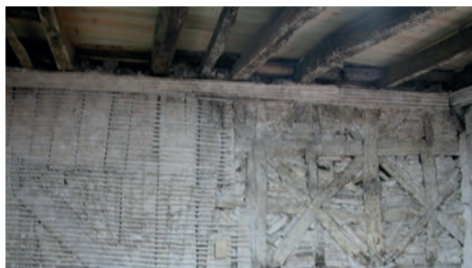
Figure 4 - "Taipa de fasquio" and "Taipa de rodízio" - Wattle and daub/Daub and half-timbered techniques in the same wall, on a traditional house in Guimarães, Portugal
