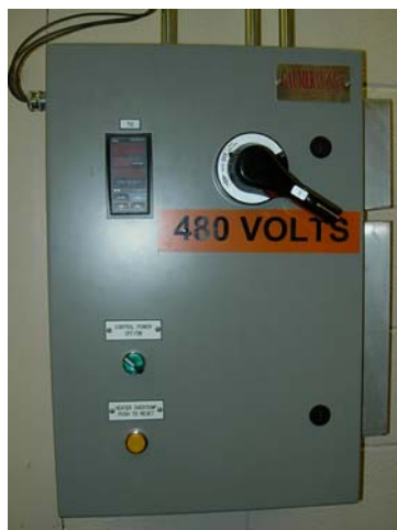
Fig. 11. Gaumer electric heater circuit breaker
