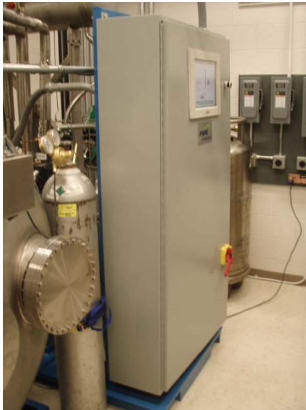
Figure IV-4: Operator Interface Enclosure
