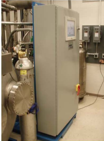
Figure 17: Operator Interface Enclosure
