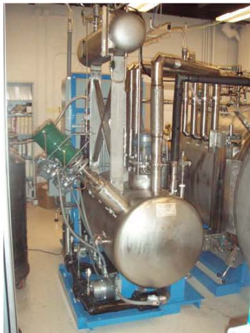
Figure 16: Thermal Control Unit (TCU)
