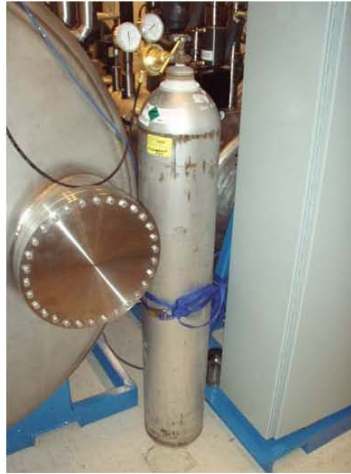
Figure 21: Gaseous Nitrogen Source
