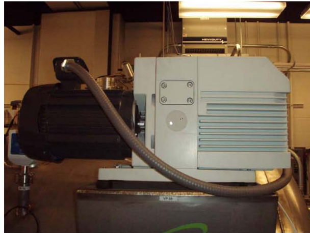
Figure 18: Roughing Pump (VP03)
