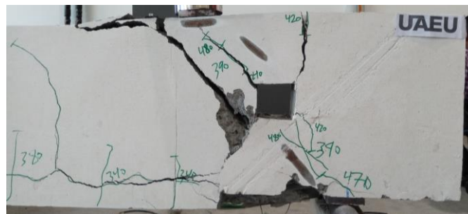
(c) close view of the crack pattern
