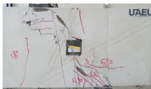
(c) close view of the crack pattern
