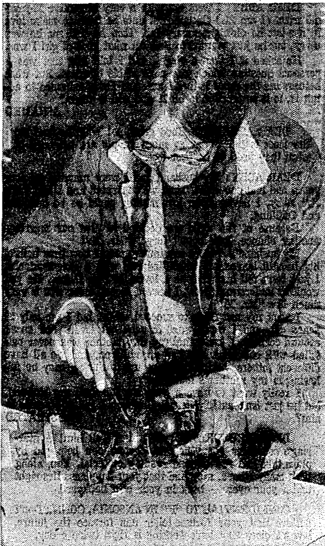
TELEPHONE REPAIR . . . Miss Gayle Orzechowski, an employee of Northwestern Bell Telephone Co., holds the rather unusual title of "combination man." She installs and repairs telephones, answers service calls and even climbs poles to repair or connect wiring. She is the first woman in the Rochester district to hold such a position. (Sunday News photos)
