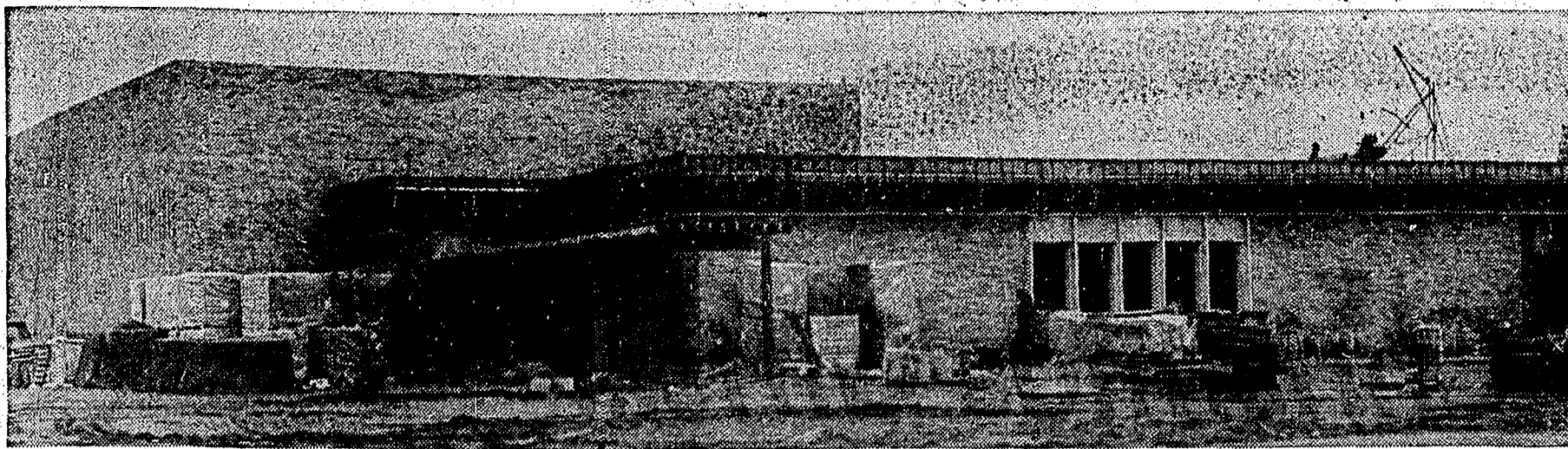
CONSTRUCTION PROGRESSING . . . Workmen continue construction on the Goodview Elementary School which is set for completion July 1. When the school opens in the fall, 250 students plus kindergarten are projected for the kindergarten through six school being built on an open space concept. The school will have three large learning centers or pods and one instructional media center, an equivalent to a combination library and audio visual room. (Sunday News photo)
