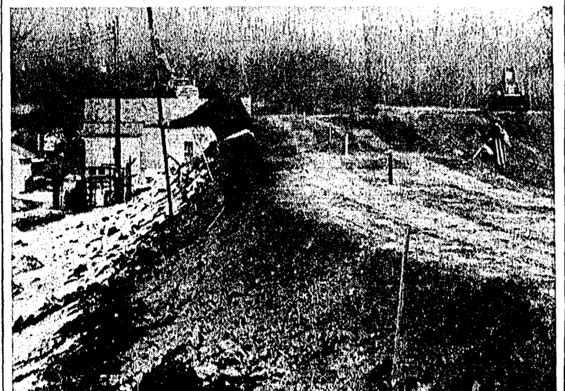
JUST CHECKING . . . Survey crew works on top of dike along Minnesota River at Chaska, Minn., Tuesday. Chaska, about 30 miles southwest of Minneapolis, is pouring tons of dirt on the dike to protect the riverfront homes from an expected record-level flood crest. The Minnesota weather bureau has predicted high water levels along the Minnesota and Mississippi River. (AP Photofax)
