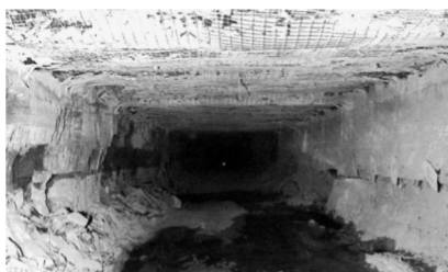
Fig. 9. Ground conditions in Entry No. 1 looking inby from the mid-pillar site prior to mining of the first panel.
