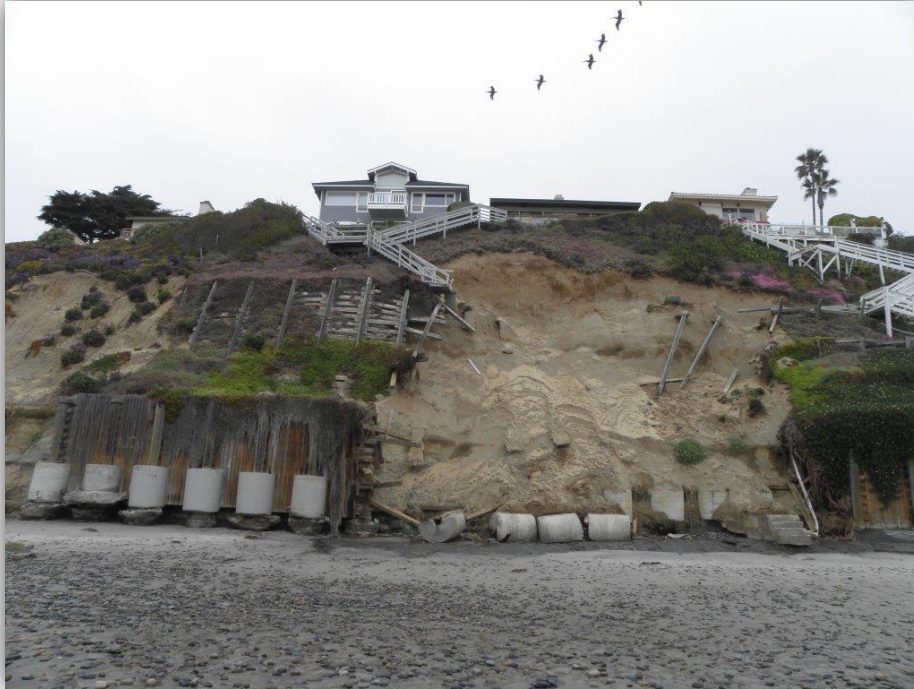
Figure 19. Photo depicting eroding bluff and exposed caissons in Encinitas, CA. (Photograph by Lesley Ewing)
