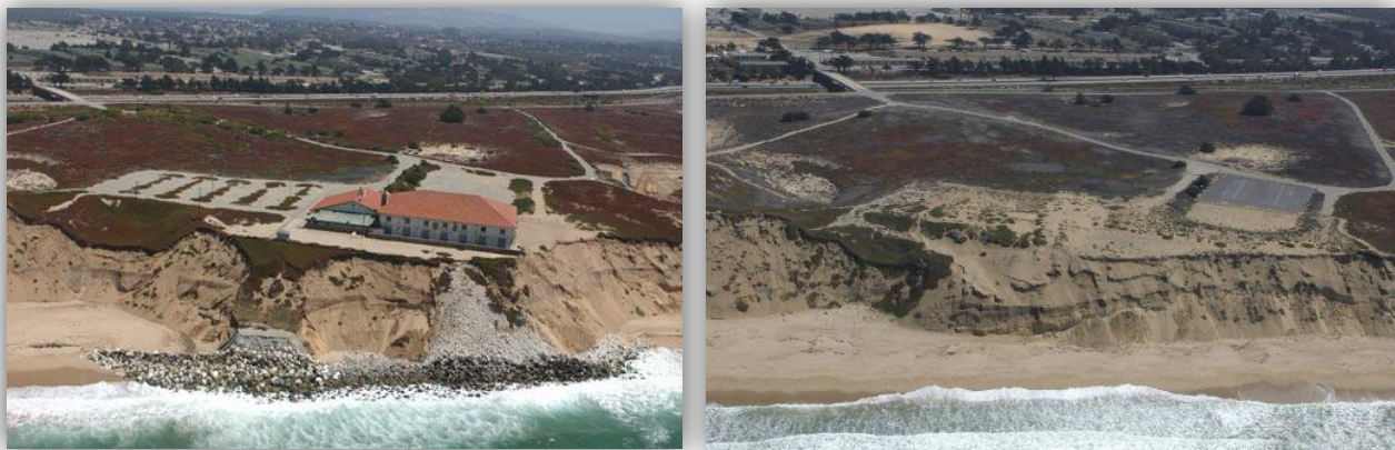
Figure 15. Photo depicting passive erosion. (Left) Passive erosion in front of a revetment at Fort Ord, illustrating the loss of beach where the development prevents the shoreline from migrating landward. The beach continues to migrate inland on either side of the revetment. (Right) Recovery of the beach following removal of the revetment and blufftop structure. (Source: California Coastal Records Project ).
