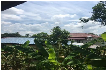
Fig. 8. (a) Adjacent rural homes with newly built roof with thicker roof sheathings did not experience any damage (b) Wind damage to interior walls and possibilities of damage to vertical support structural system when the roof was breached
