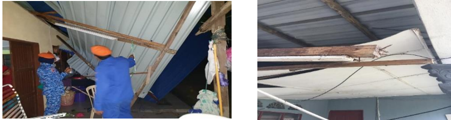
Fig. 4. (a) Roof sheathing damage due to overturning failure mode at roof edges and absence of cross bracing; Post Restricted Use and barricade the side of the house (b) Weak and rusted nail connections
