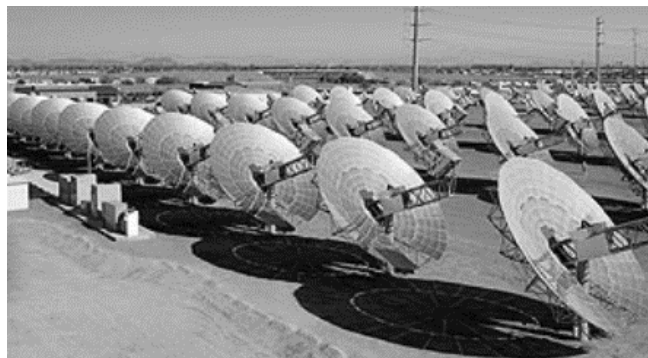
Figure 16. Maricopa Solar Project, Arizona. Source: Tessera Solar.
