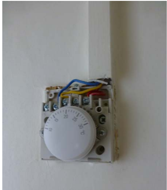
Fig. 1 A new well-established room thermostat
