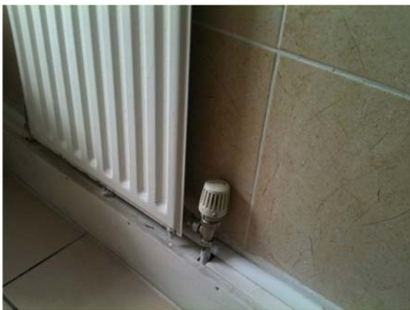
Fig. 4 Radiators 'locked in' by boxed away pipes
