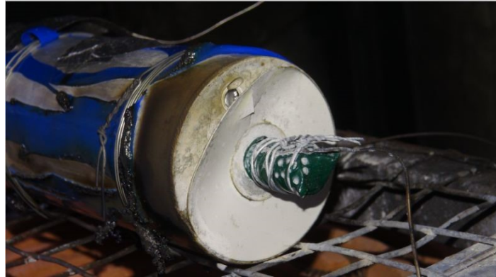
Fig. 4 The safety vent near the collector column
