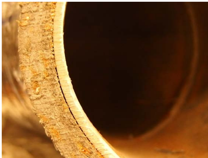
Fig. 7: De-bonding of the CFRP from the pipe elbow surface.
