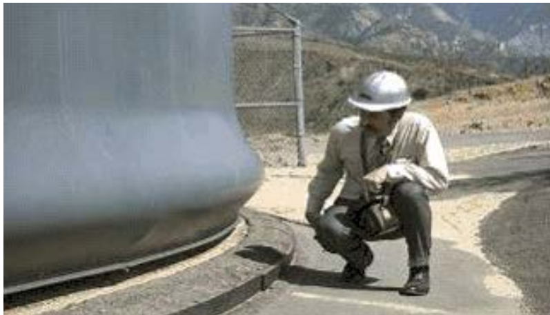
Figure 1: Elephant's foot buckling in liquid storage tanks [39].
