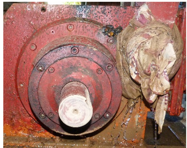
Fig. 3. Leakage from a turbine casing.
