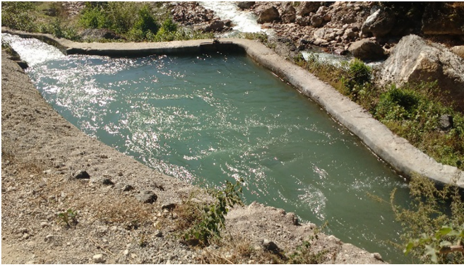
Fig. 4. Ineffective shape of de-silting bay.
