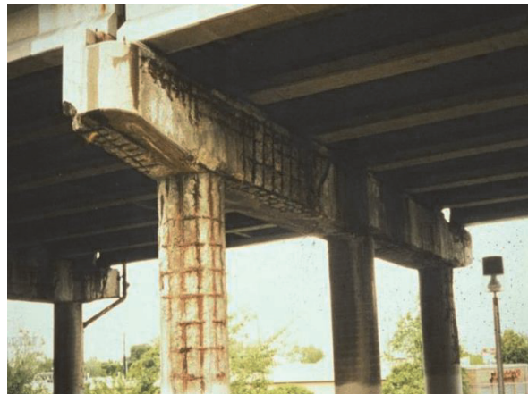
Figure 19. Concrete piers of reinforced steel with corrosion problems [18].
