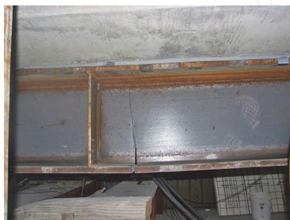
Figure 22. Steel beam with fatigue crack failure [21].
