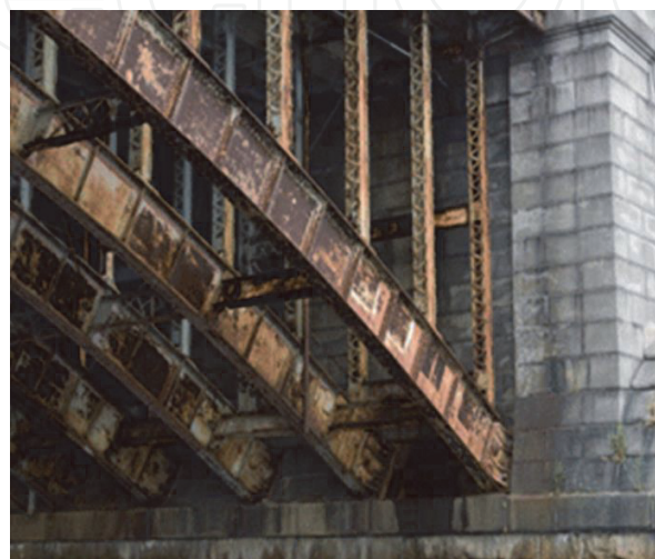
Figure 20. Bridge of structural steel with corrosion problems [19].
