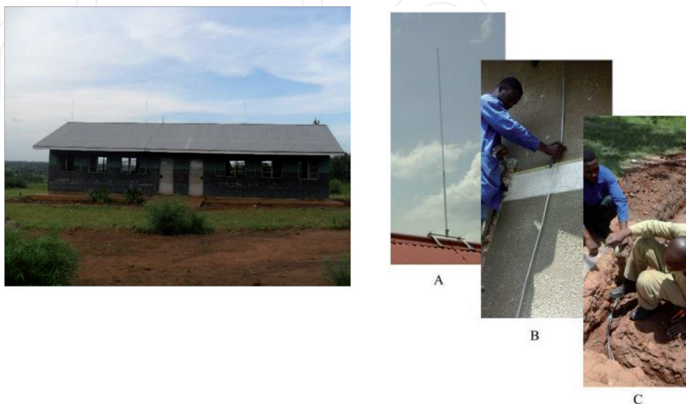
Figure 10. Installation of lightning protection system at a typical classroom building at Runyanya school, Uganda. Details: (A) air terminal; (B) down conductor; and (C) ground terminal or "earthing ring." (©ACLENet).
