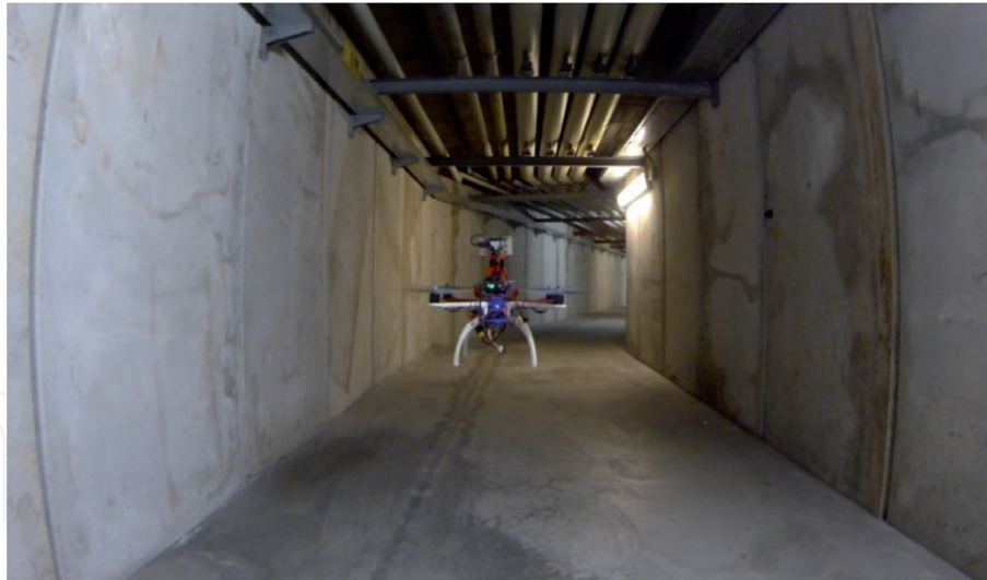
Figure 11. Tunnel inspection performed by the UAV during the test of system validation.
