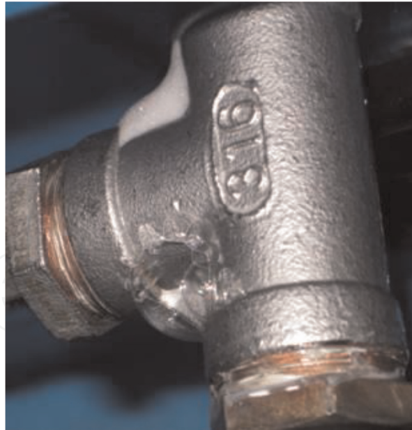
Figure 22. Source of leakage identified after on-site inspection.
