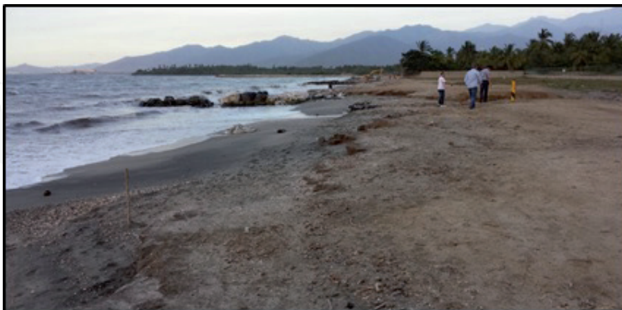
Figure 21. Severe beach erosion along the Costa Verde Cienega coast, exposing a crucial pipeline (yellow marker). Note the low-profile sandbag groin and the earth-moving machine at the top of the picture. The earth-moving machine was moving sand from the upland to nourish the beach and attempting to control the erosion.
