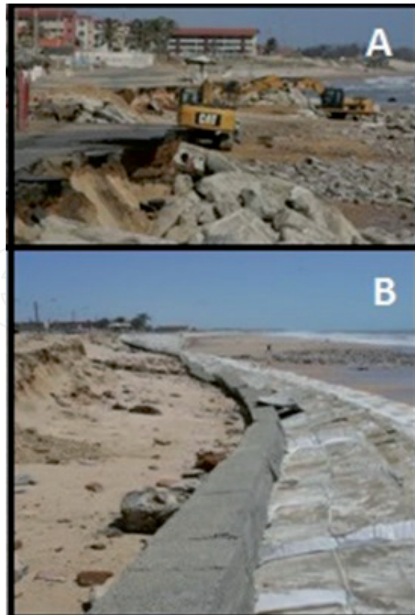
Figure 6. (A) Erosion in Icarai Beach, 25 km downdrift of Mucuripe harbor, resulting from the interventions in Fortaleza city and in the area around the harbor. The rising of the sea must also be a factor producing the erosion. (B) Bag-wall installed in Icarai Beach in the 2010s, already destroyed by the waves.
