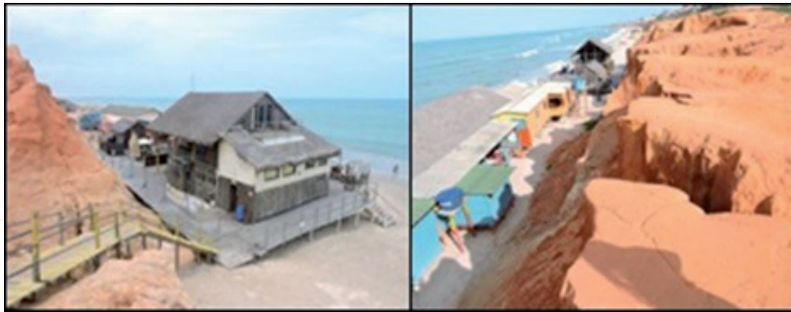
Figure 12. Tourist equipment installed very close to the unstable sea cliffs, running the risk of being buried by landslides.
